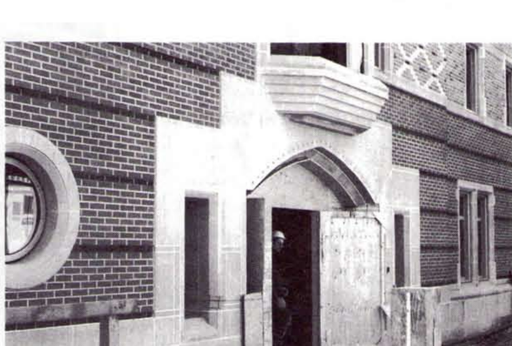
To maintain continuity with the sanctuary, the church's new administrative wing will feature limestone in a variety of applications.
