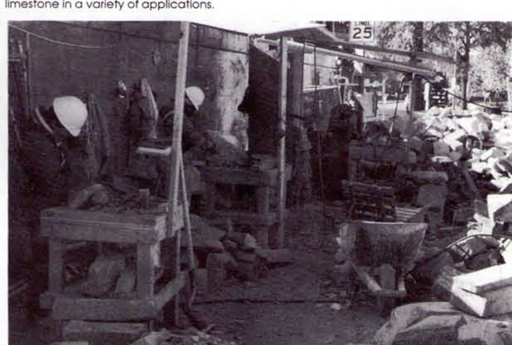
Much of the church's stone cladding is being handworked on the job site.
