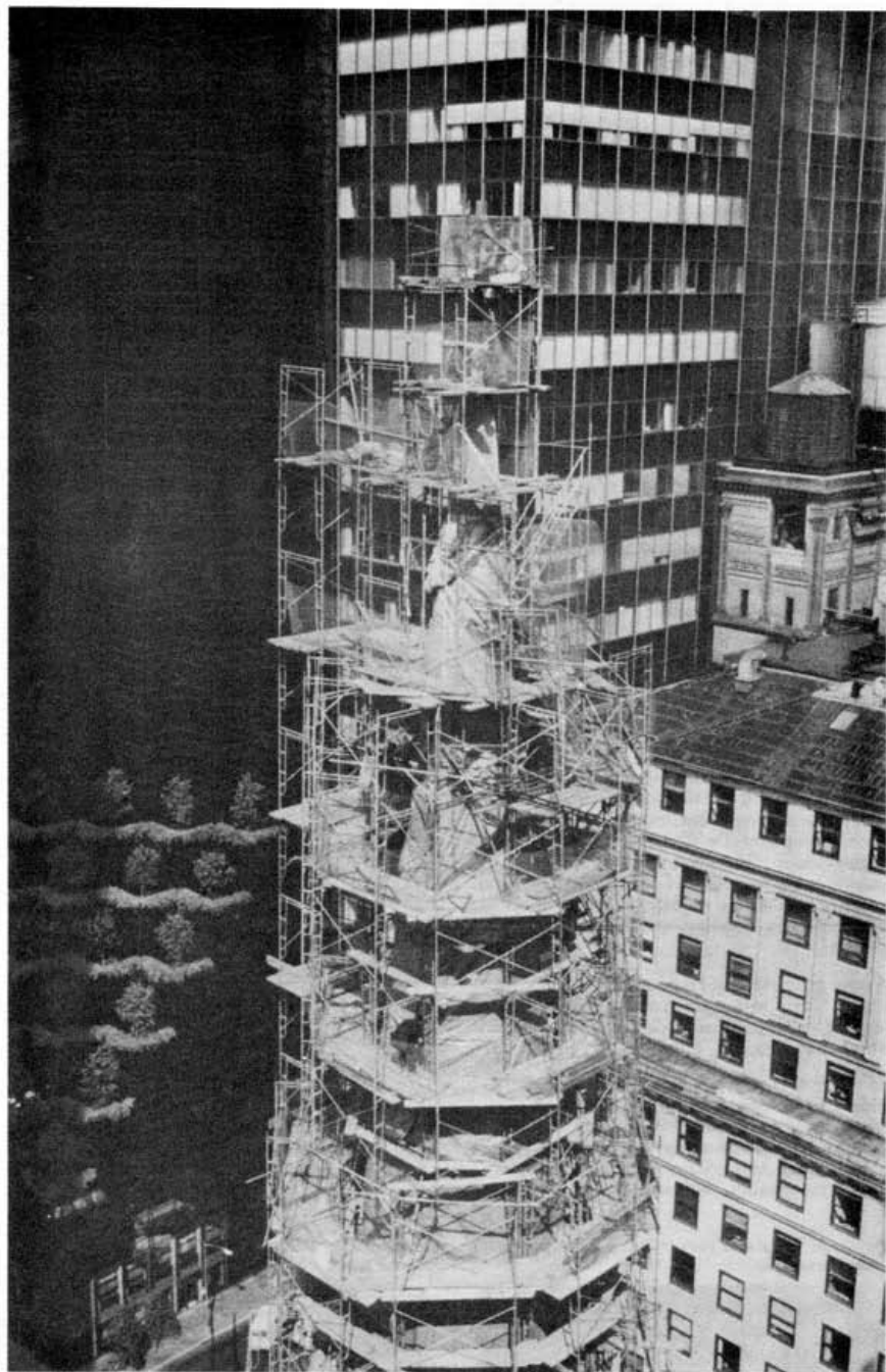
Gilding the cross atop Fifth Avenue Presbyterian Church. Cathedral Stoneworks is the principal contractor for the $3.5 million "stone-by-stone" restoration.
